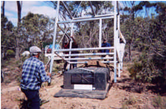
Bill Bennell supervising installation of the new toilet block at Mt Ridley Reserve.
